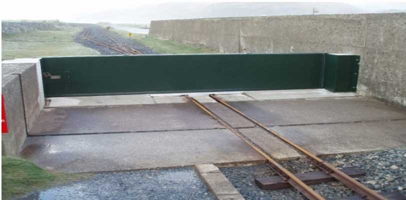
Flood gate closed as precaution
